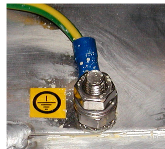
Place of connection of the earthing wire
